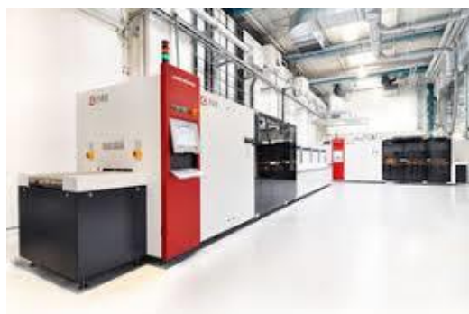
Figure 7. Drying & Sintering Furnace Equipment
